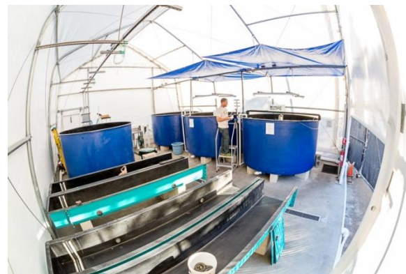
Figure 2. – New larval production facility with self-cleaning rearing tanks and halibut raceways.
